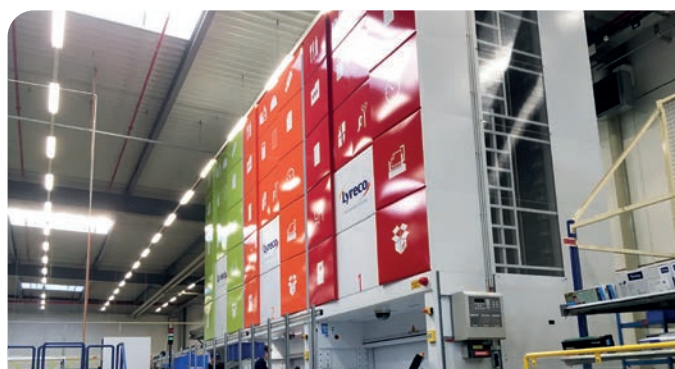
Fire protection system integration
